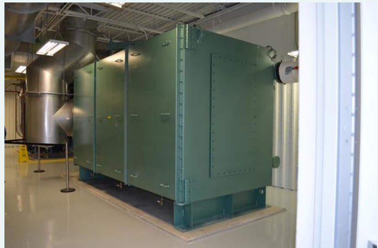
CCHP- Heat Exchanger
