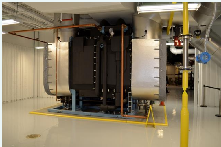
CCHP-Gas Absorption Chiller
